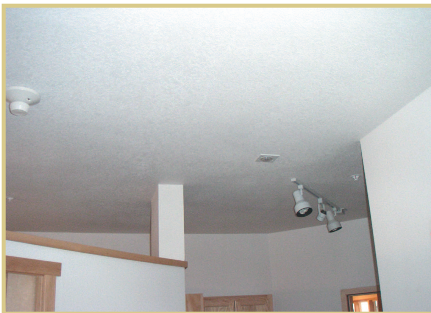
Figure 1. A typical view of a resident's ceiling, which includes a smoke alarm, IR sensor, sprinkler heads, and track lighting. All rooms also have monitoring switches on doors and stationary movement sensors. Although some features, such as the track lights, have wall switches, they are controlled through programmable logic controllers.
